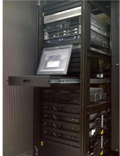
Fig. 4.5 : Rack mounted servers
