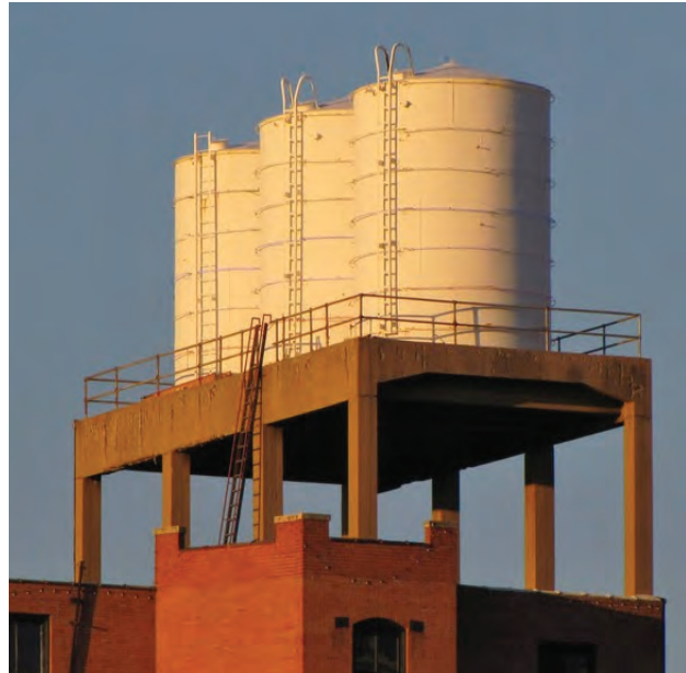
Overhead water tanks
